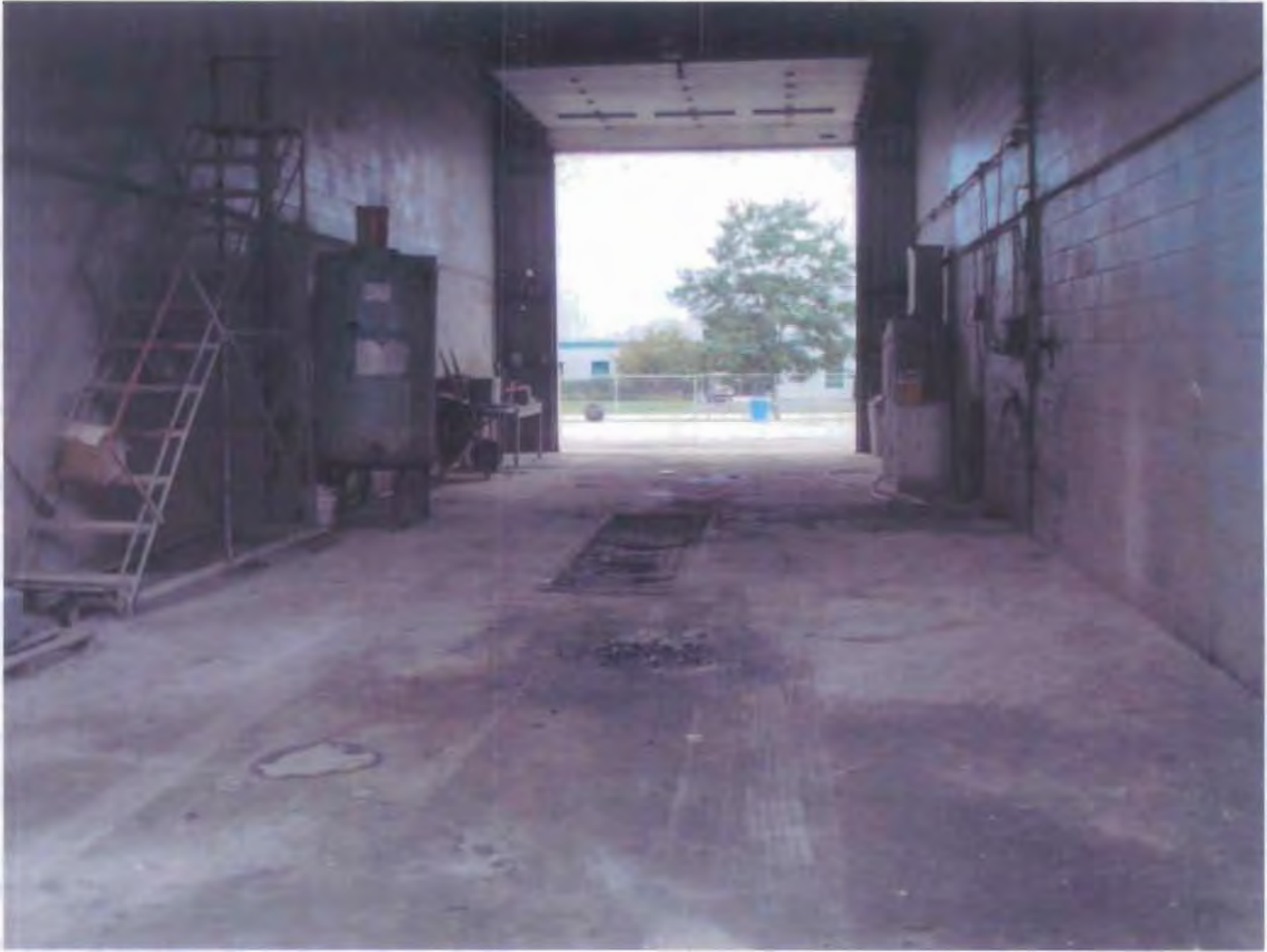
Photo 2 - Enclosed truck washing area, with triple basin, which also discharges to the same storm sewer as in previous photo.
