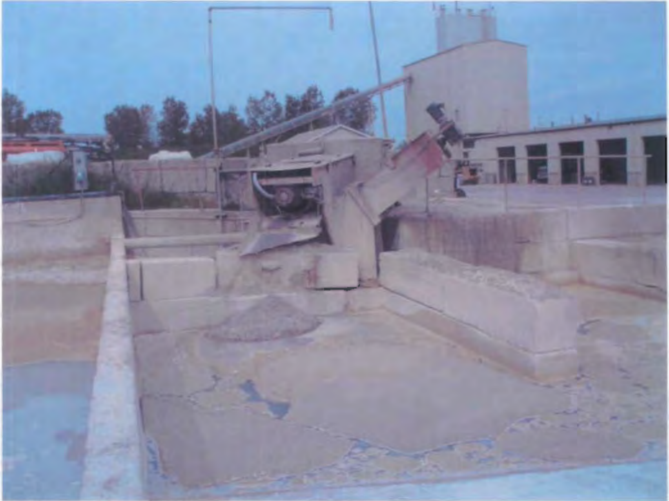
Photo 4 – Another component of the concrete washout area. Note concrete filling station and truck bays in background.
