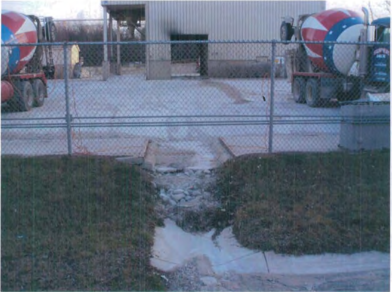
Photo 1 – Runoff from the fill house is draining directly to the road ditch. There is also a lot of process material in the road ditch.
