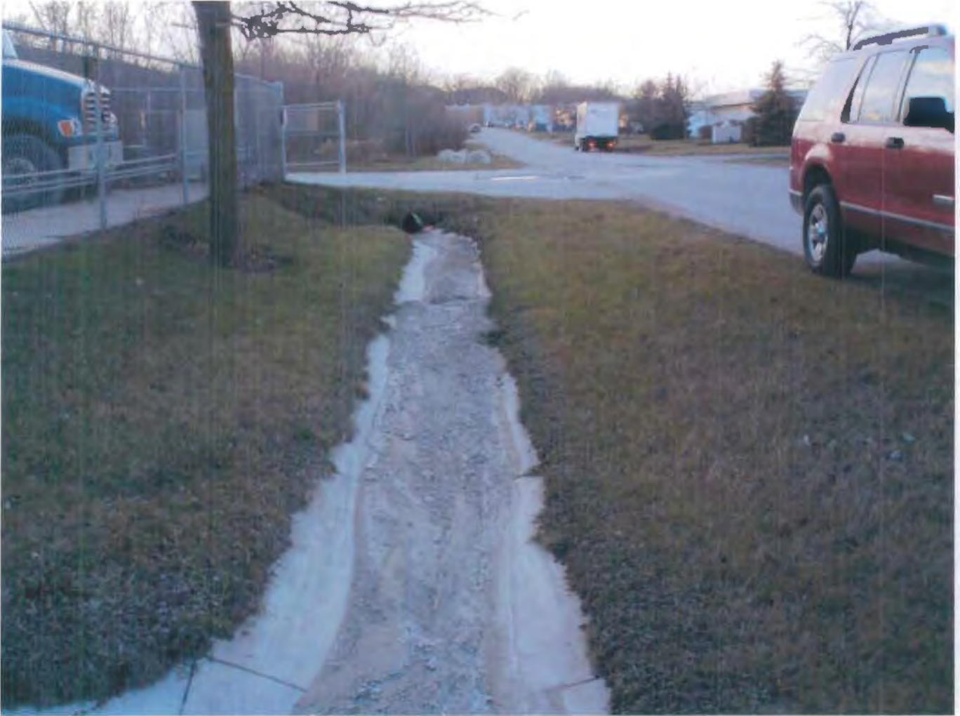
Photo 2 – View of the front road ditch with collected process material
