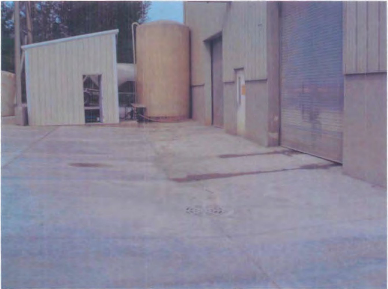
Photo 1 – Unprotected storm sewer in back of concrete filling station
