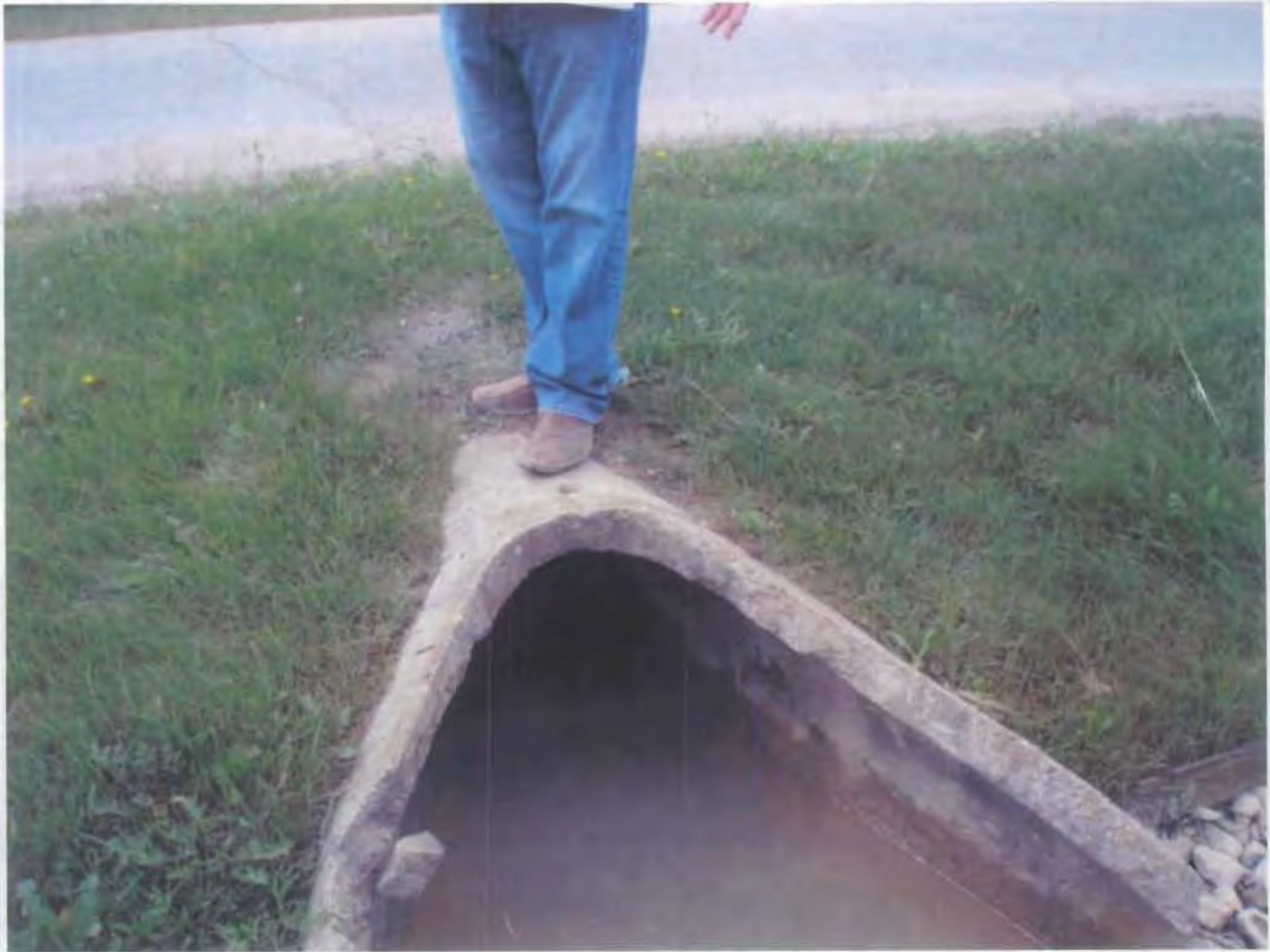
Photo 10 – This is the culvert where storm water flows from the south side of the street to the north side of the street and into the storm ditch, shown in Photo 9. Note the water quality and color are similar to the settling pond shown in Photo 8.
