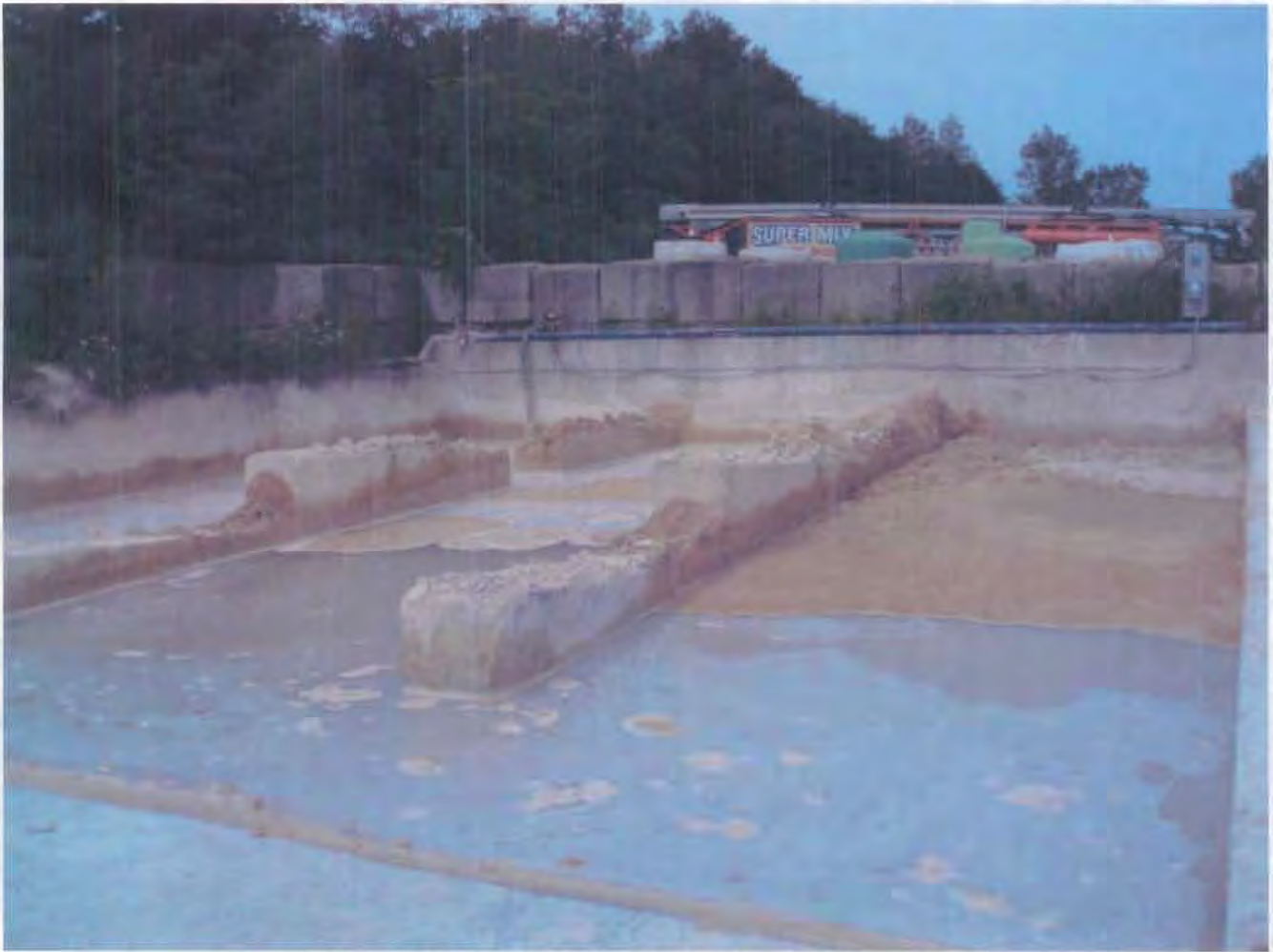
Photo 3 - Concrete settling basin in back of property where washout is supposed to occur.
