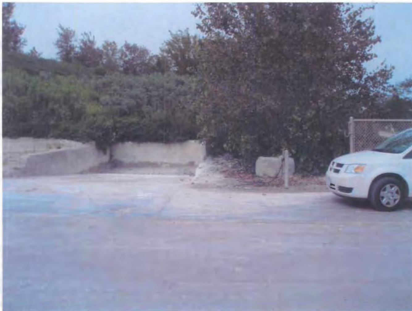
Photo 6 - This is the area near the front entrance where some washout had been occurring. Note that the area around the pump that was supposed to be abandoned is wet.
