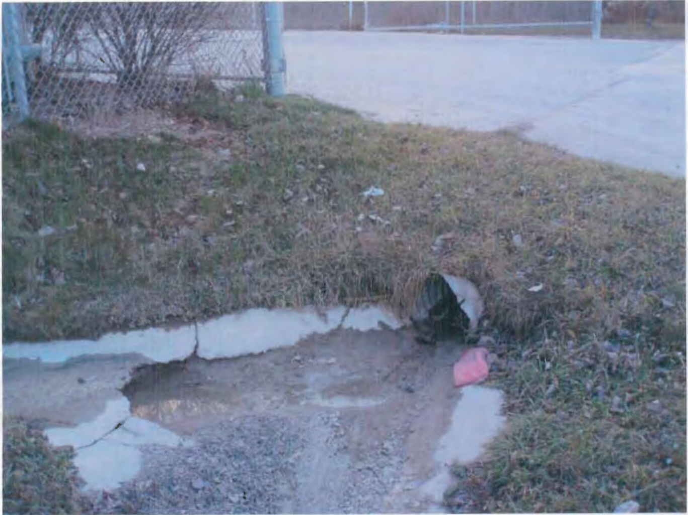
Photo 3 – Culvert by driveway entrance to the facility, showing collected process material. Note also contaminated side stream that enters here as well.
